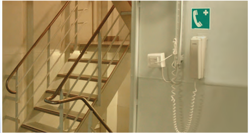
4392C (Emergency telephone)
