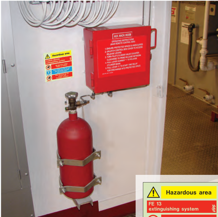
6516E (Hazardous area, carbon dioxide extinguishing system)
