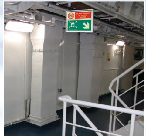
8190PT (Do not obstruct or restrict access)
